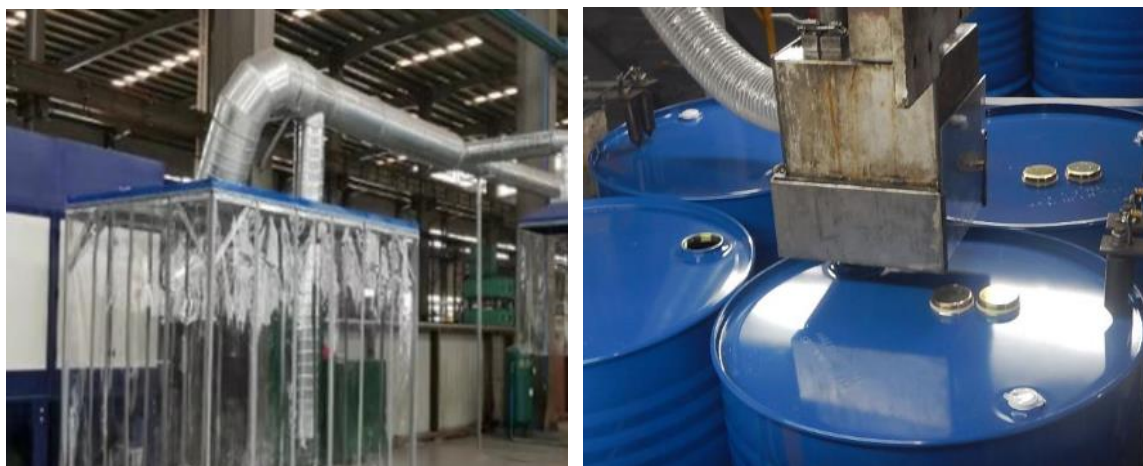
封闭+集气罩抽风
