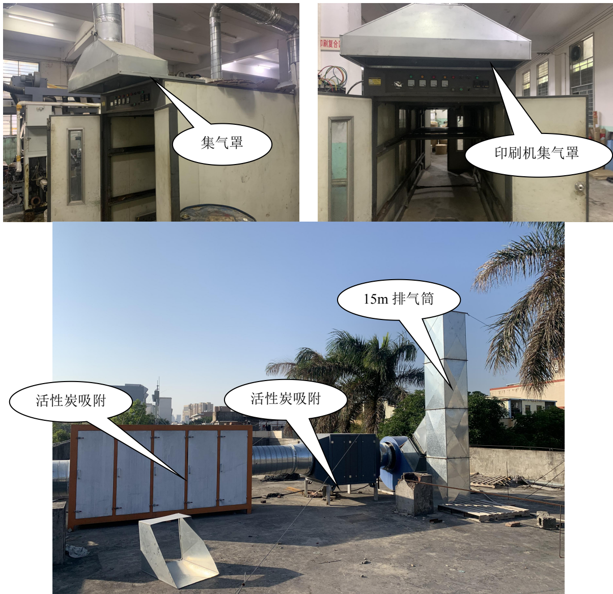
有机废气：集气罩+活性炭吸附+15m 排气筒
