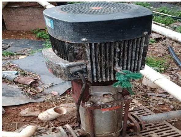
灌溉水输送高压水泵
