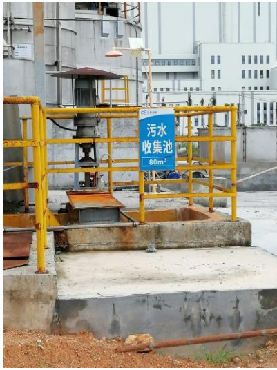
硅胶废水收集池 (1×80m 3 )
