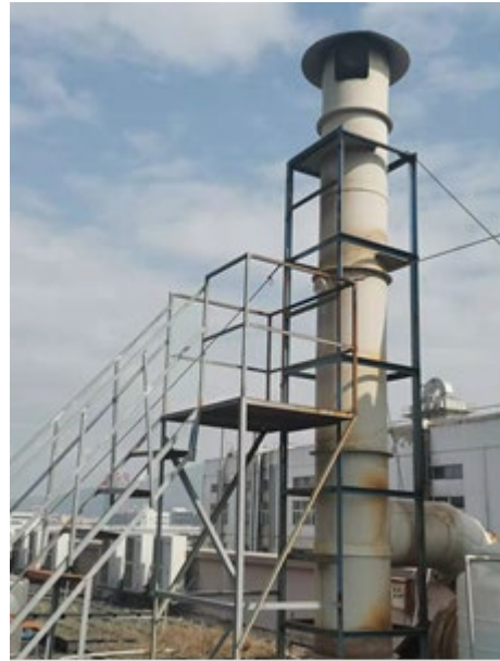
酸性废气洗涤塔设施、排气筒 (FQ-202218-1)
