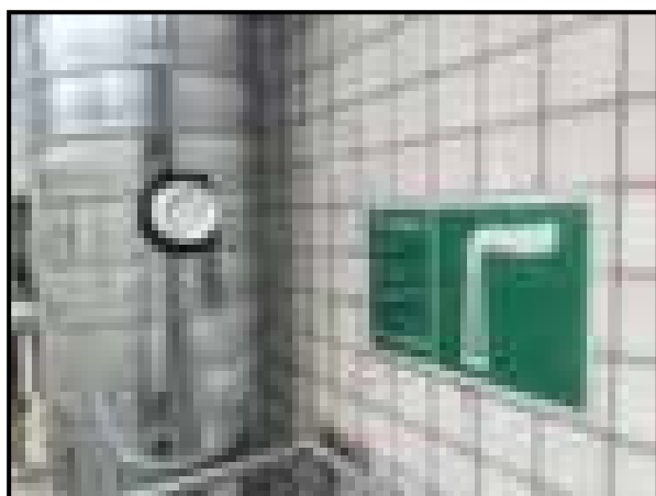
废气排放口监测孔和标识
