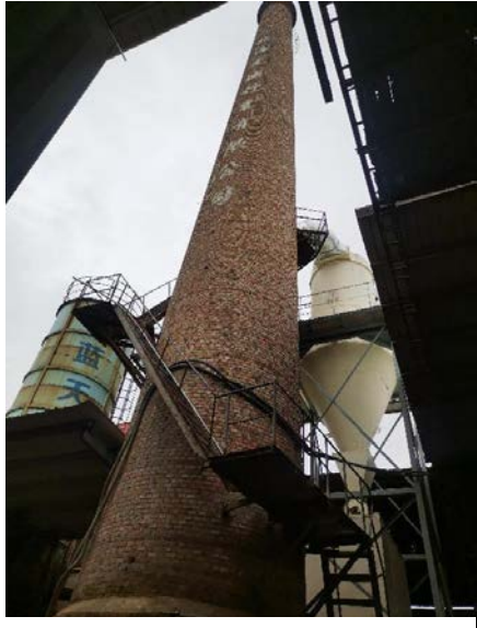
DA001 破碎粉尘排气筒
